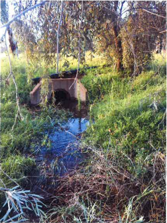
Photo 10: The northeast sediment pond discharged during 2022, was sampled and was compliant with EPA discharge limits for the site. Photo taken 8 January 2022.
