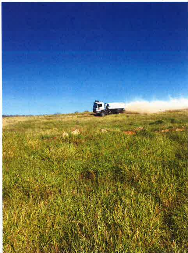
Photo 20: Agricultural lime being spread at a rate of 2t/Ha on the top of heap leach final landform in April 2021.
