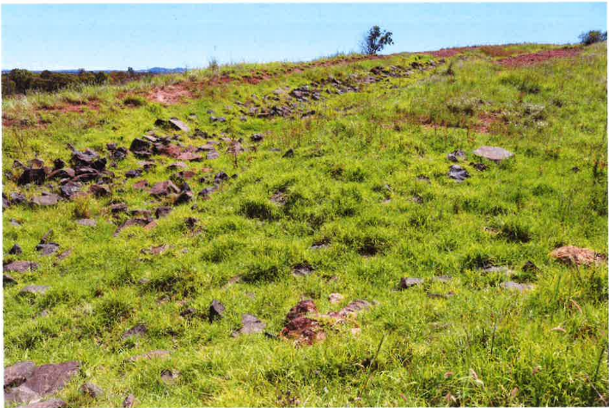
Photo 12: Rock-lined flume designed and built by Soil Con in 2005. Kikuyu grass thrives between basalt rock/blocks. This single flume sheds water from the heap leach landform.
