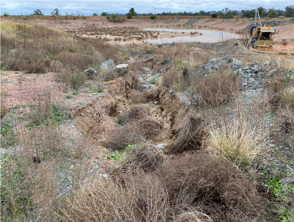
Photo 7 – Erosion near the WRE 3 drop structure leading to SD2
