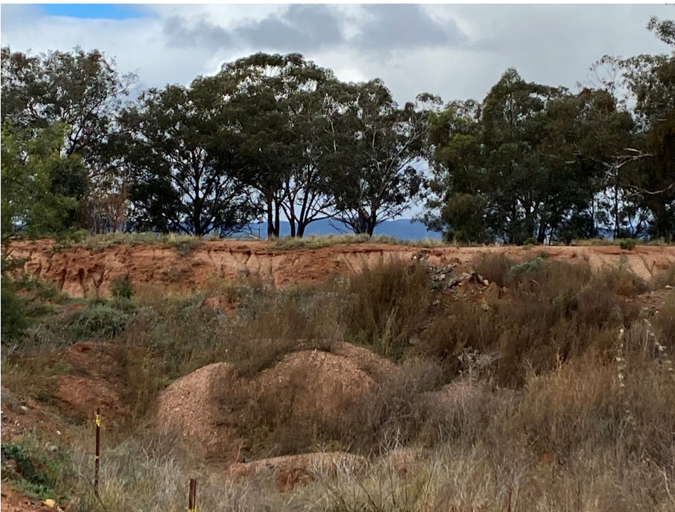
Photo 4 – Some bunds at site have rill erosion due to dispersive soils
