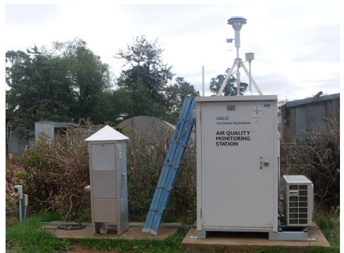
Air quality monitoring station
