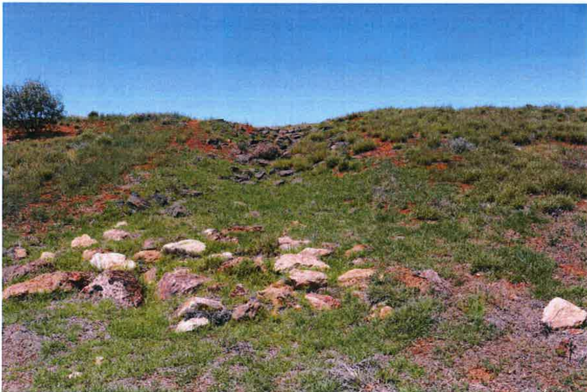
A well-functioning rock-lined drop structure on heap leach landform. Photo taken 17 December 2018.
