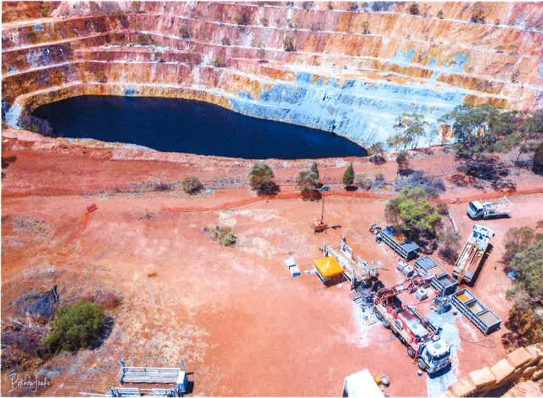
Diamond drilling program 2018-2019 testing gold resources below the Proprietary pit. Photo courtesy of Mitchell taken 13 Feb 2019.
