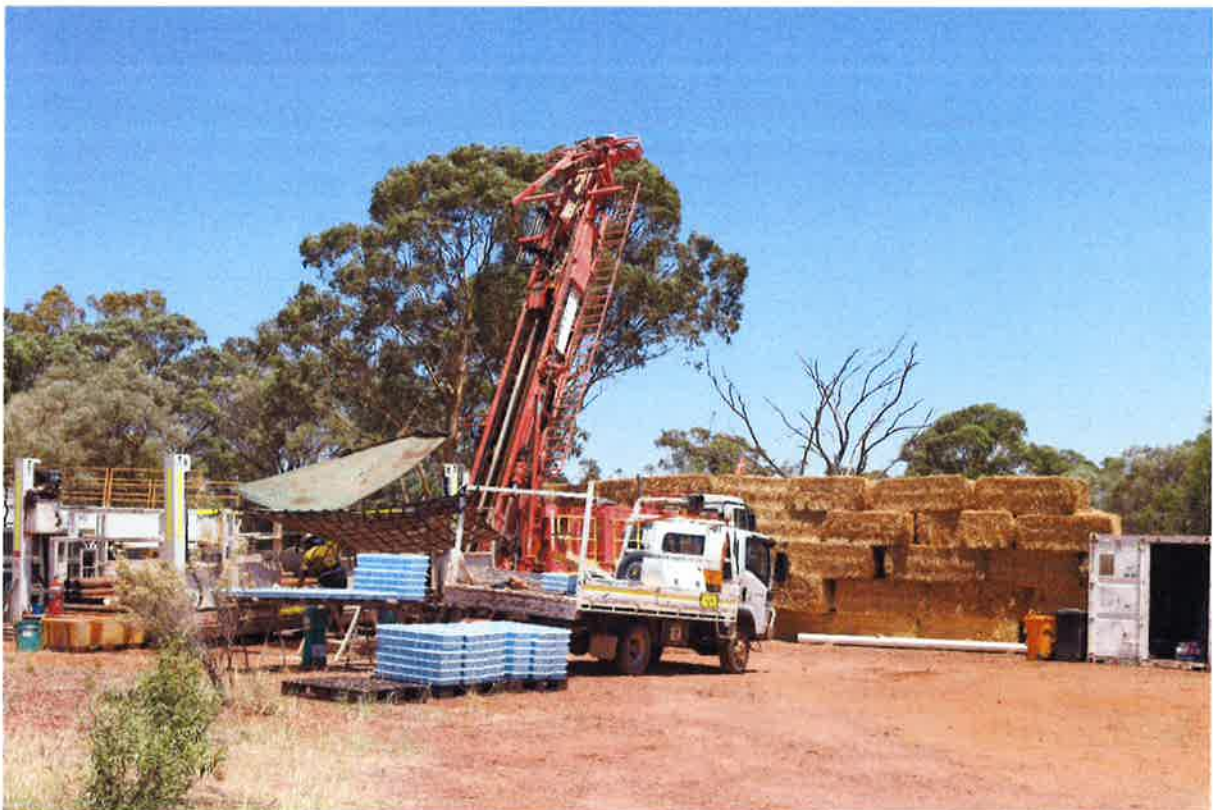
Diamond drilling behind a sound wall of hay bales. Photo taken 8 February 2019.
