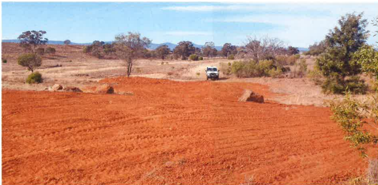
ROM pad re-topsoiling of an area that once held a stockpile of sulphidic material. The sulphides were removed to Parkers Pit (toe of Gilligan's island). Photo taken 29 July 2019.
