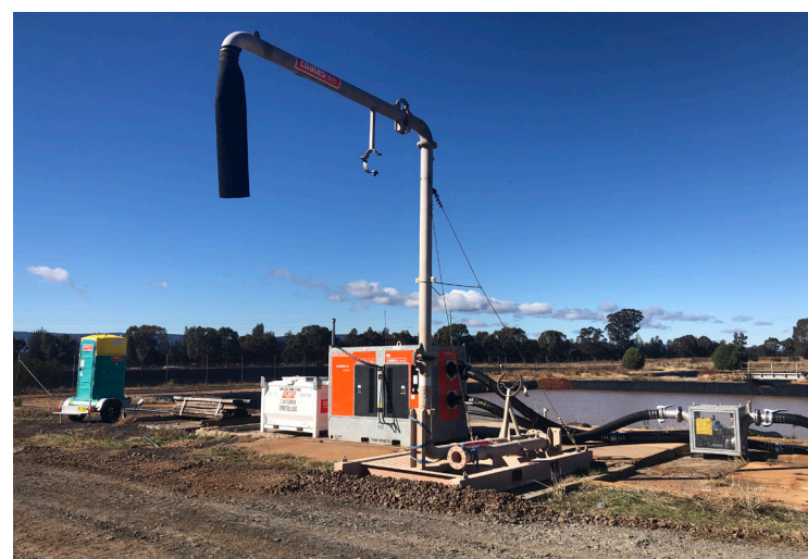
Temporary pumping infrastructure used to fill water tankers at Peak Hill Gold Mine.
