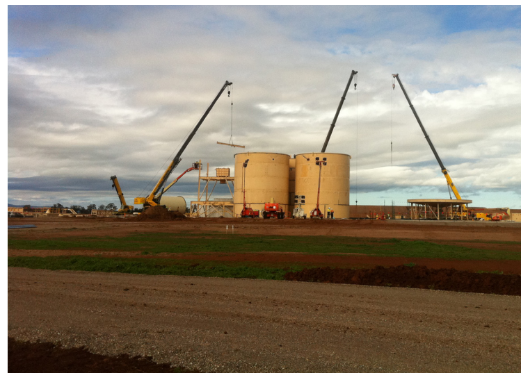
First three carbon in-leach (CIL) towers in position
