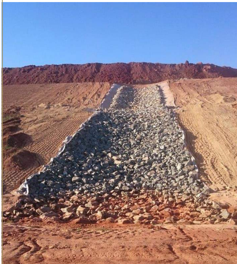
Rehabilitation: Drainage channels go in prior to treating topsoil and sowing pasture vegetation
