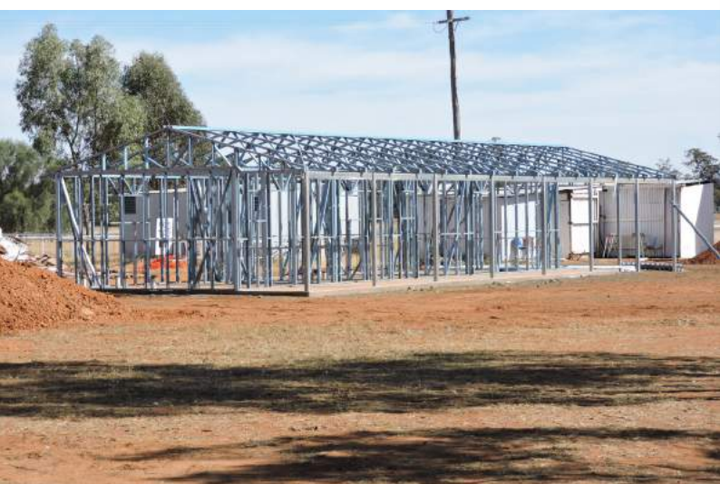
Construction of new amenities building is underway at the Tomingley Sport and Recreation Ground
