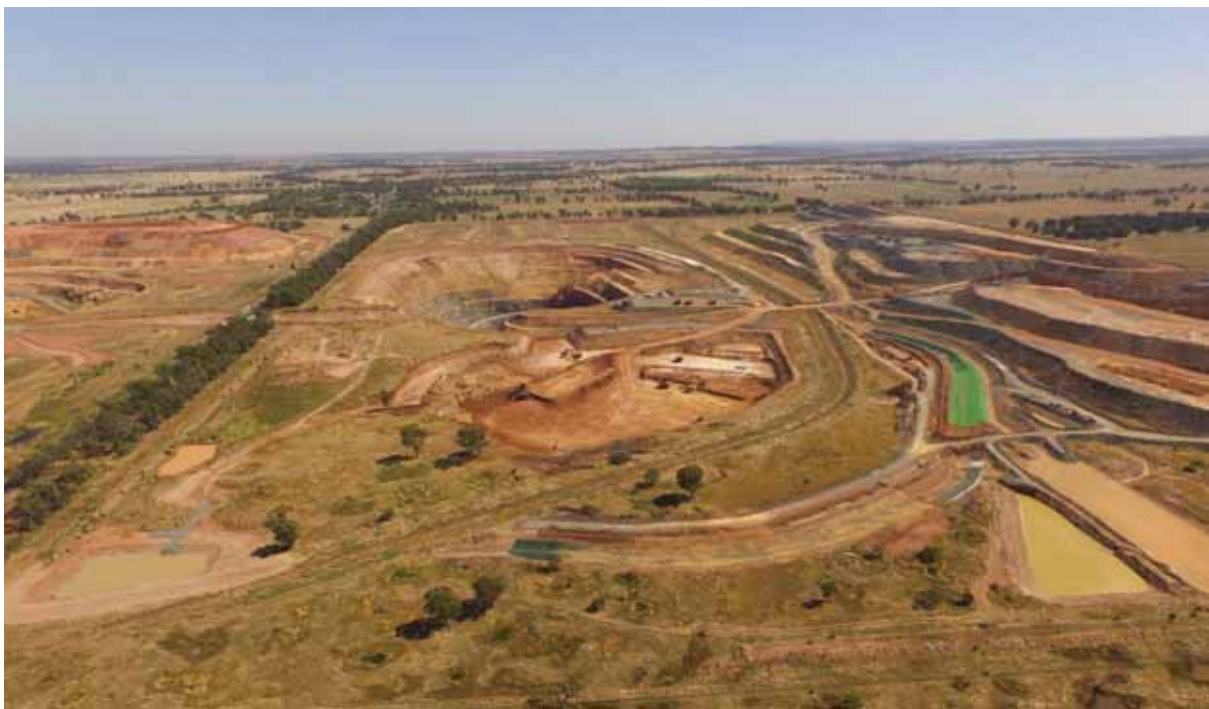
Plate 5: Works to re-align Caloma Central Drain, enlarge Sediment Basin SP4 and construct Sediment Basin SP7.
